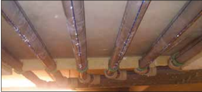
Illustration 6.5 Condensation on cold water lines
