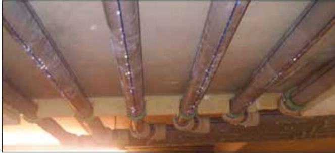
Illustration 6.5 Condensation on cold water lines
