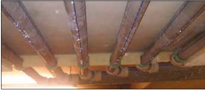
Illustration 6.5 Condensation on cold water lines
