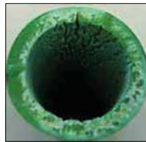
Illustration 3.7 Damage observed with not properly stabilized PP-R under extreme conditions
